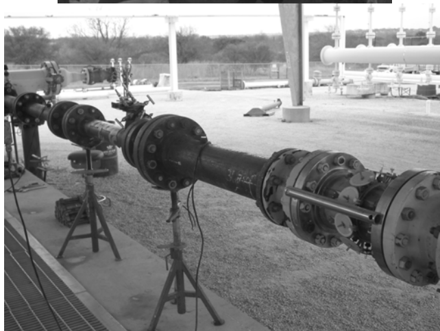
Figure A-12. Multi-hole Pitot tube used to confirm swirl angle in Non-Standard Test 3, shown up close, at left, and downstream of swirl generator device, at right.
